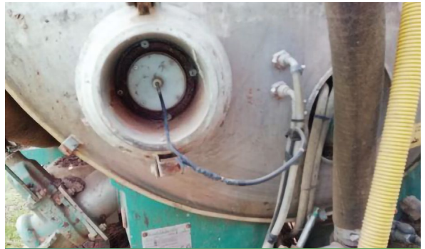
Conductivity meter installed in the transport tank
