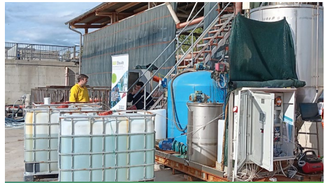
Pilot treatment plant for struvite recovering from digestate
